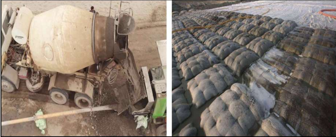
Fig.- 6- (a) Image showing the process of concrete filling (b) Image showing installed Articulating Grouted Concrete Mattress after concrete filling
